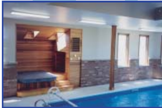
Pool water heating, pool dehumidification, pool air conditioning, pool area heating. Virgil, Ontario
