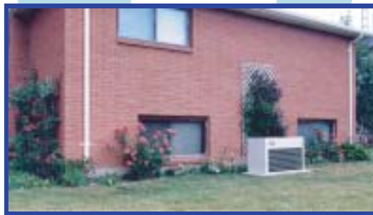
Ductless heating and cooling 10 rooms. Welland, Ontario
