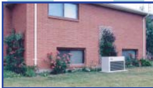
Ductless heating and cooling 10 rooms. Welland, Ontario
