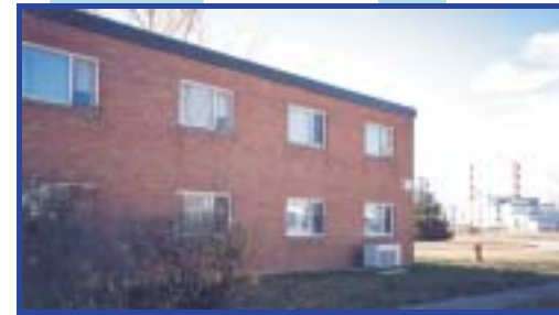
Ductless air conditioning. Military Academy, Ottawa, Ontario
